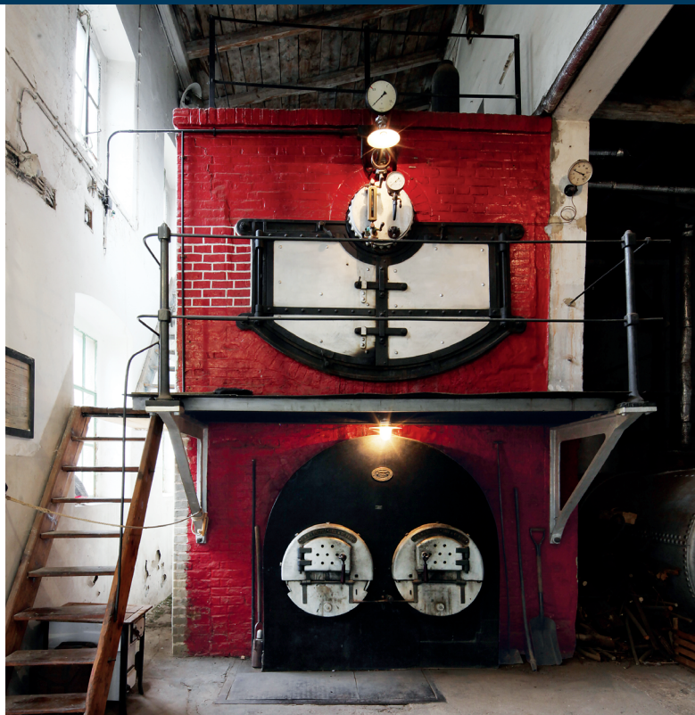
Breitfeld, Daněk & Co. steam boiler from 1907, 2025
